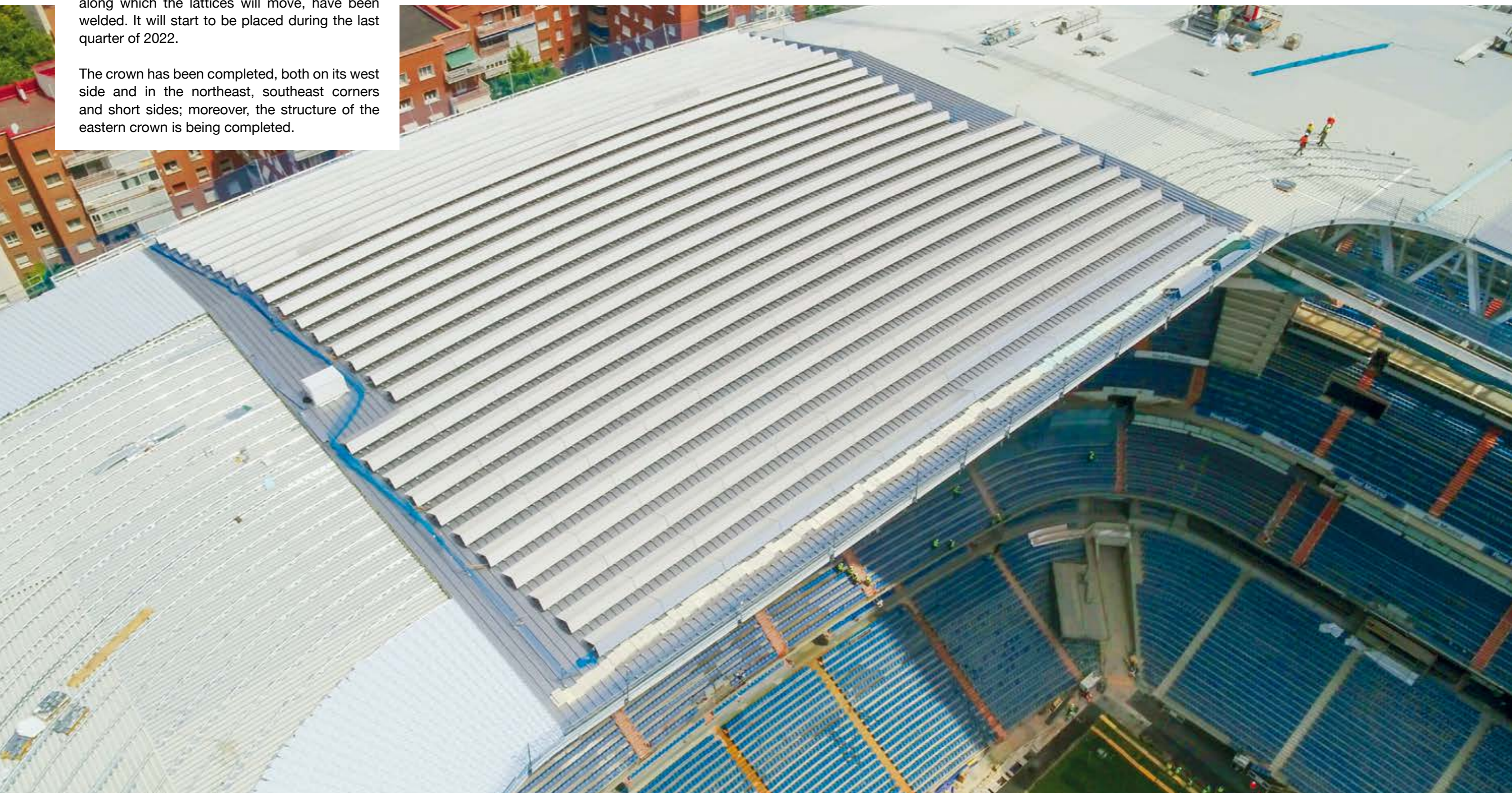
After the completion of the beams and the covering elements, stainless steel slats are now being placed on the roof.
